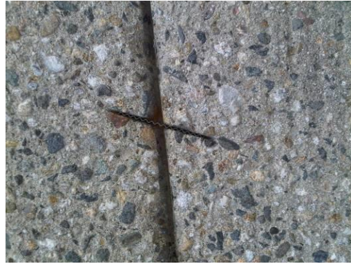
Joints are cramped
