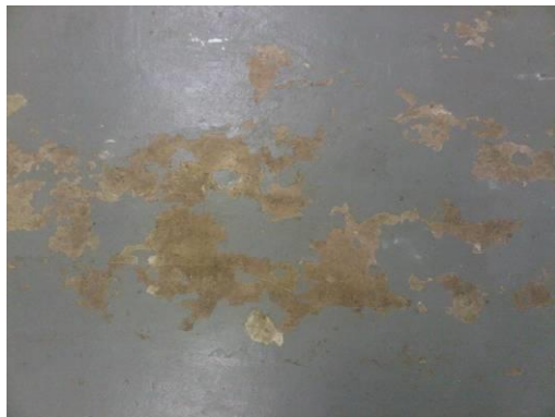
The old EP coating is peeling off
