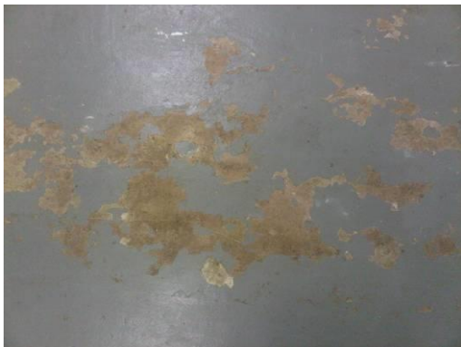
The old EP paint is spalling
