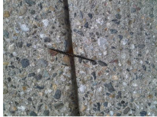
Joints are cramped
