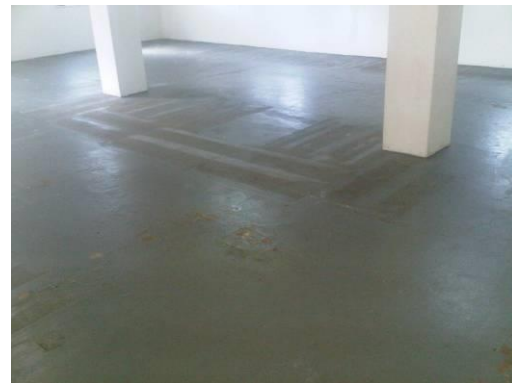
The existent floor is uneven
