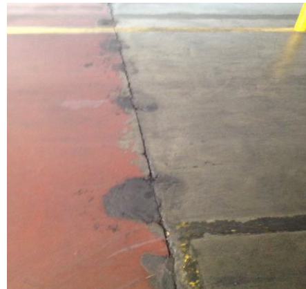
Joints are broken.
