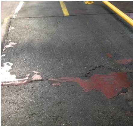
The floors are uneven.
