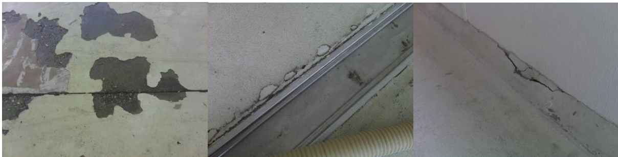
EP coating is spalling
