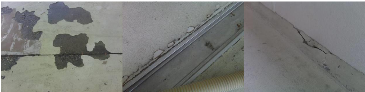
EP coating is spalling
