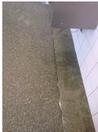
old concrete was not easy to clean
