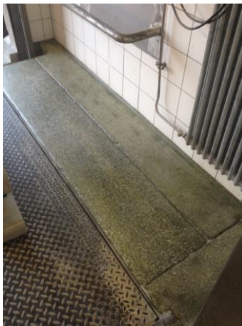
The old floor with cracks
