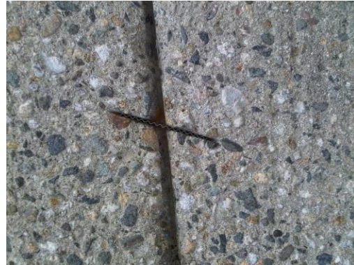
Joints are cramped
